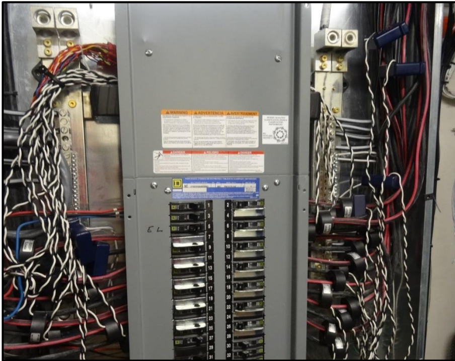
Figure C - 1: Current Transformers Connected to the HOBBO Logger
