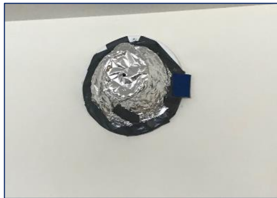
Figure 17: Unit 3 - Air Supply Inlet
