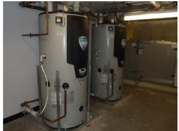
Figure 34: Condensing Water Heaters that Provide Space Heating and DHW to the Building
