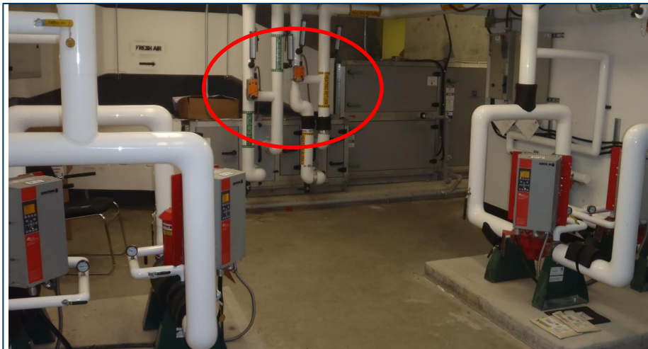
Figure E - 3: Heating and Cooling Pump and Three-way Valves (Ref. to red circle)
