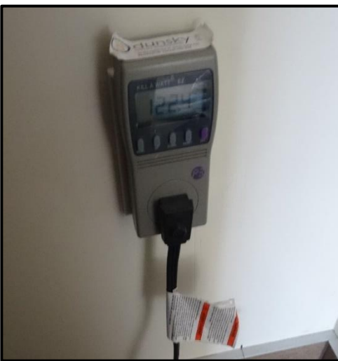
Figure C - 5: Kill-a-Watt (installed in the common kitchen)
