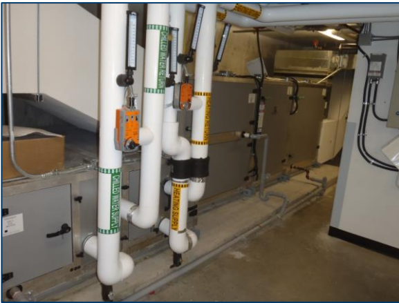
Figure E - 1: ERV Serving the Building
