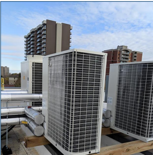
Figure E - 4: Air Cooled Chillers – New Units (2x) in Front, Existing Unit (back)
