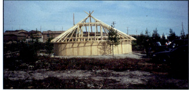
Traditional dwelling under construction in the cultural village beside the new community.
