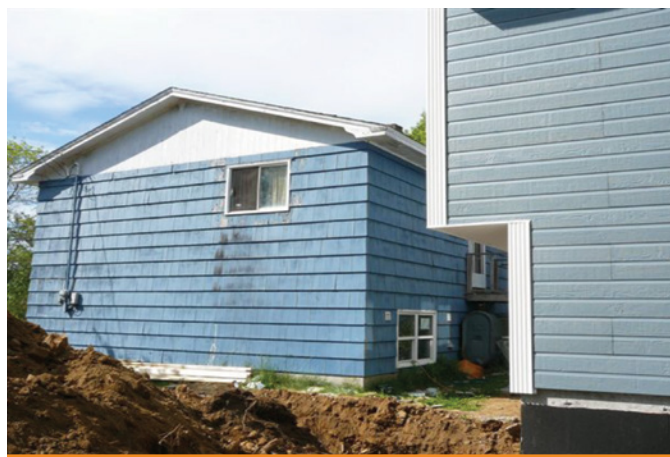
Figure 2 The house on the left had a history of leak problems and lack of maintenance. It is being replaced by the house on the right
