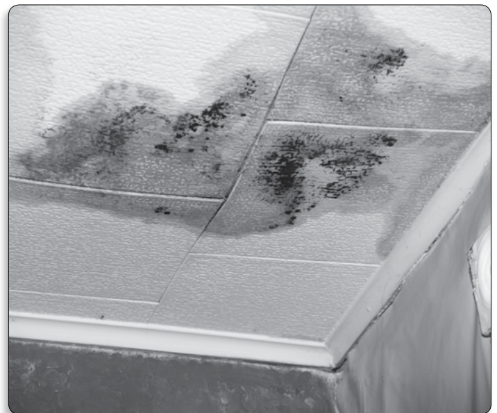
Water staining and mould growth on ceiling tiles
