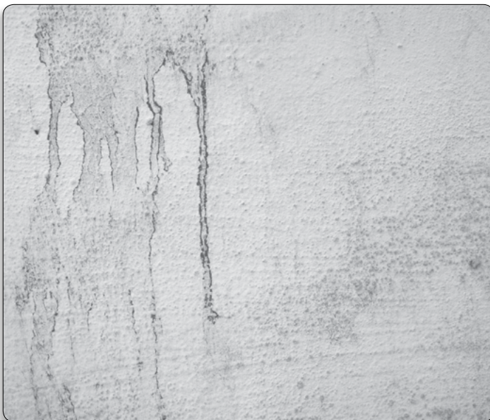
Stains on materials often indicate water damage
