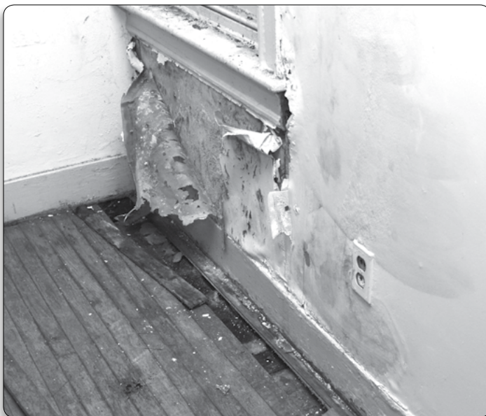
Water damage under a window
