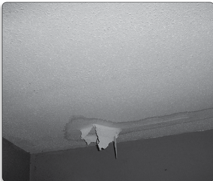
Water damage on a ceiling
